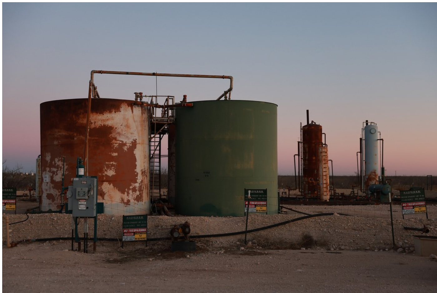
Storage tanks that are part of a system for holding wastewater and crude oil are seen in the Permian Basin region of Texas. Joe Raedle/Getty Images
