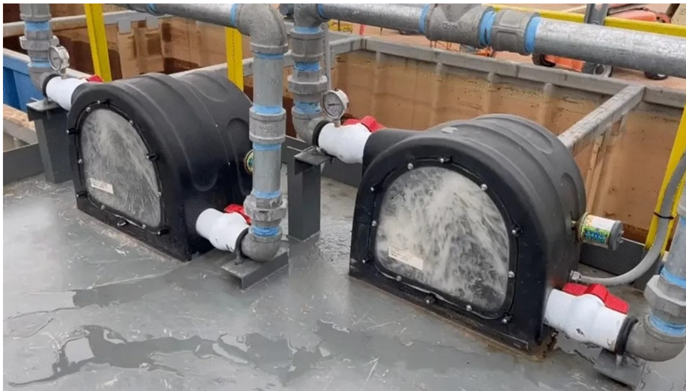
Water drives a pair of turbines at the Starr County test site. (Sage Geosystems)
