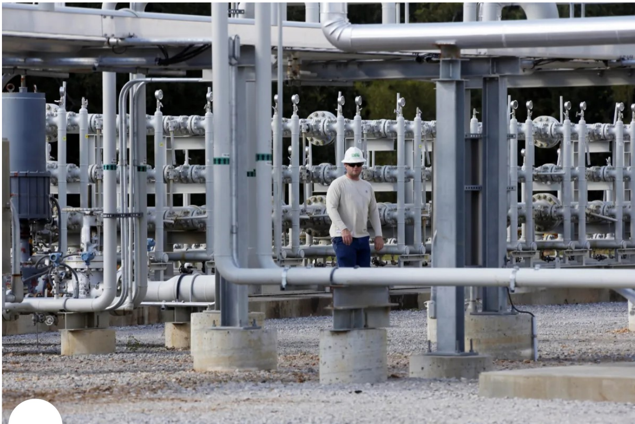
In a photo taken Oct. 22, 2013, a worker walks past a CO2 manifold at Denbury Resources Inc.'s, Tinsley Facility in Tinsley, Miss. Denbury Resources hopes to bring new life to old oil fields by pumping in carbon dioxide to force additional oil to the surface. (AP Photo/Rogelio V. Solis)
