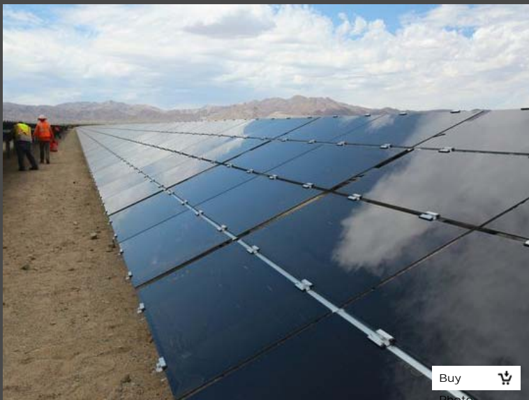
Workers build the 550-megawatt Desert Sunlight solar farm in Desert Center, about an hour east of the Coachella Valley, on Aug. 20, 2014. (Photo: Crystal Chatham/The Desert Sun)
