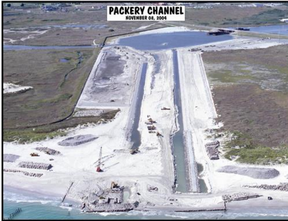
Figure 2. Construction at Packery Channel, November 8, 2004. Photo courtesy of the City of Corpus Christi ( http://www.cctexas.edu/engineering/packery ).
