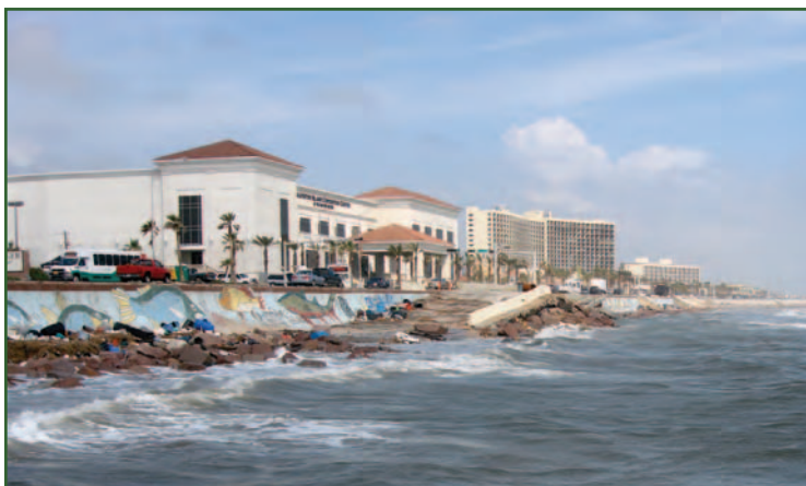
The Galveston Seawall after Hurricane Ike and before restoration.
