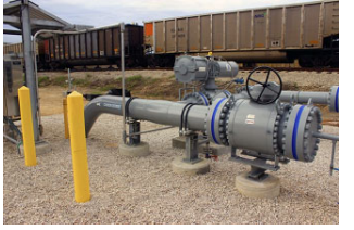
Pipe carrying supercritical carbon dioxide goes into the ground, headed for the West Ranch oil field 80 miles away. (Photo courtesy of NRG Energy)
