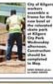
City of Kilgore workers are visible in the background at the construction site for the new branch of the Citizens National Bank in Kilgore. Construction should be completed by May 2017.
