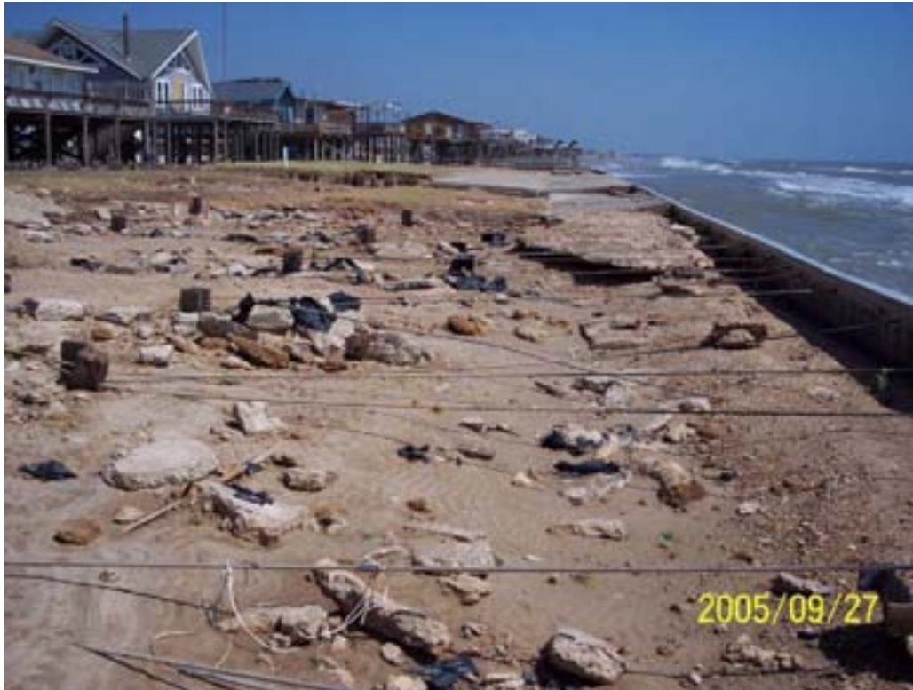
Figure 9. Damaged southwest bulkhead in Surfside Beach.
