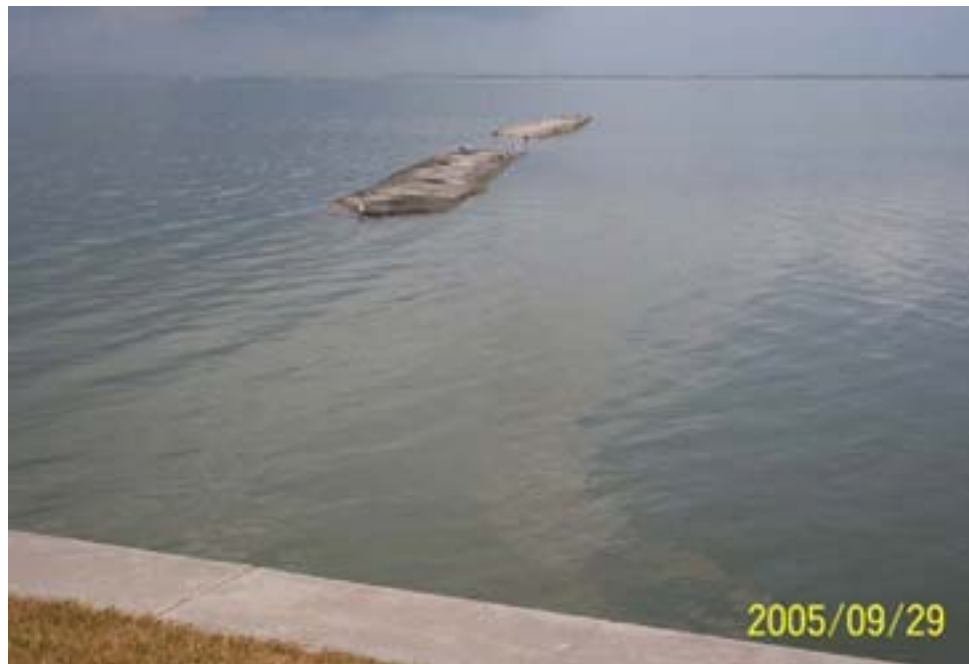
Figure 34. Damaged geotextile tube protecting marsh restoration project adjacent to Jamaica Beach (Galveston Island State Park project). The UV shroud is not present, the tube appears slumped and flattened. It is possible that the tube was damaged further during Hurricane Rita.
