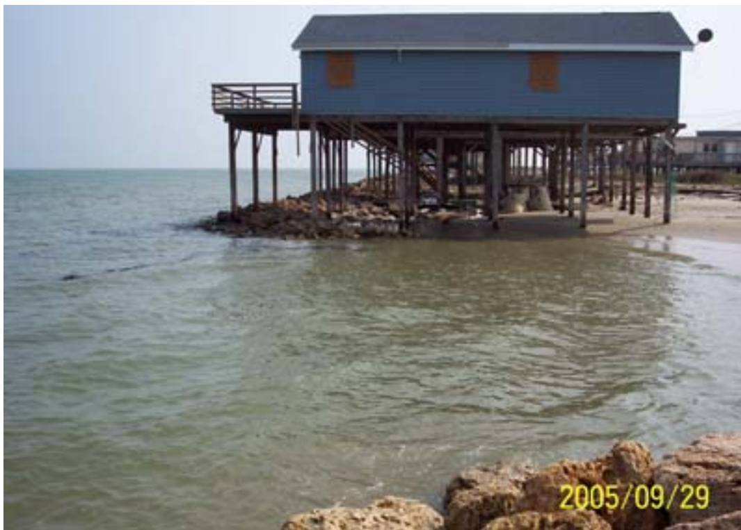
Figure 21. Houses in surf zone in Treasure Island subdivision. Remnants of geotextile tube in water on left. Tube was largely destroyed before Rita.
