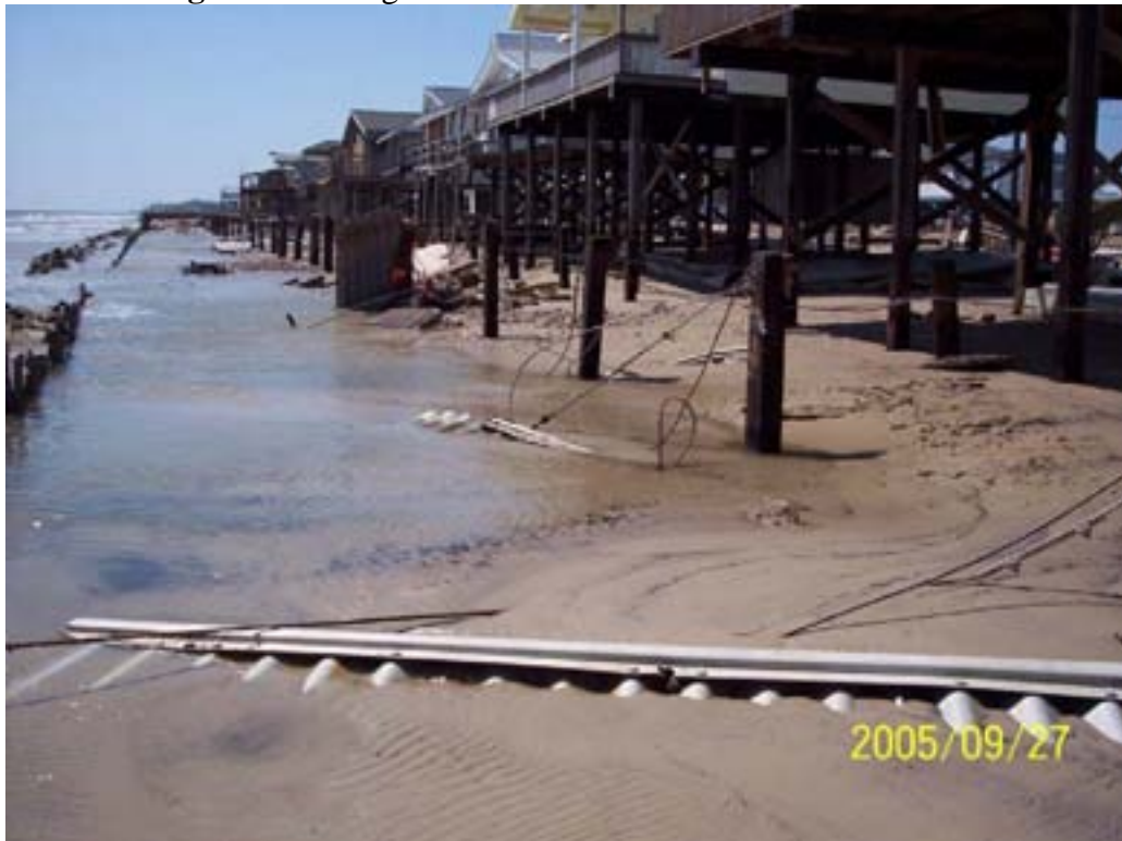
Figure 10. Destroyed northeast bulkhead in Surfside Beach.
