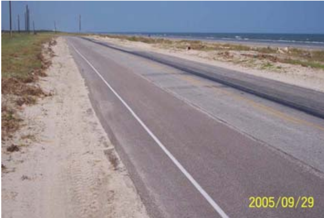
Figure 16. Follets Island. The road is only about 50 m from the shoreline here and had no pre-storm foredune. Sand was transported onto the road by Rita's waves and surge and then bulldozed.
