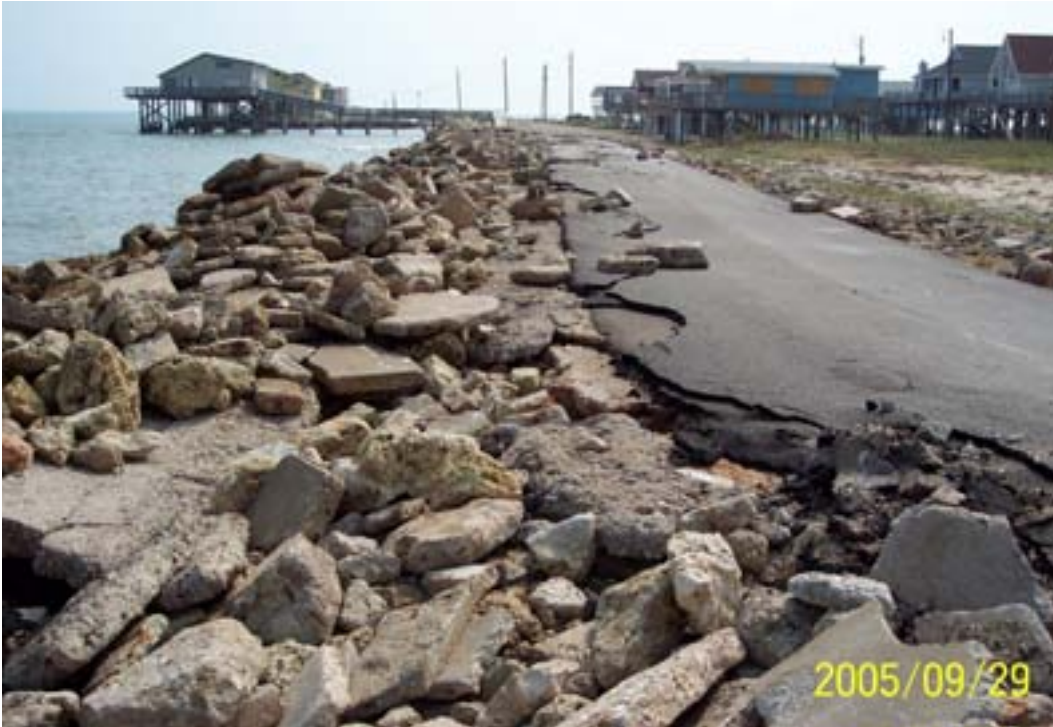
Figure 18. Treasure Island subdivision. Asphalt road is damaged and rip rap dislodged.
