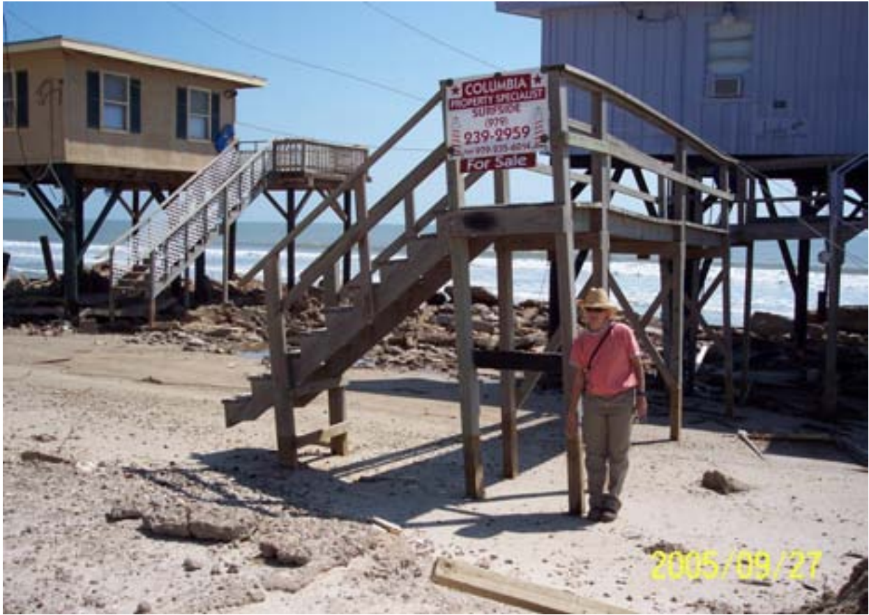
Figure 8. Erosion exposing stair supports indicating a lowering of the beach in Surfside Beach.
