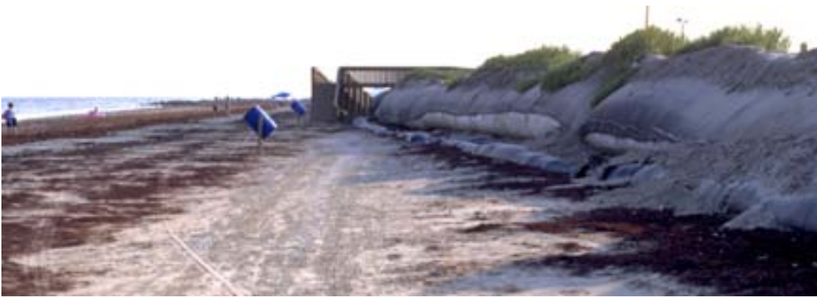
Figure 7. Example of fully exposed geotextile tube front and scour apron at the Dellanera project on Galveston Island, July 18, 2001.
