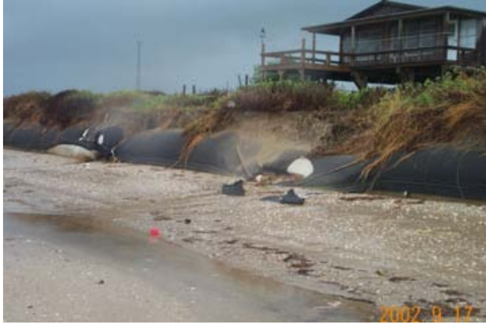
Figure 24. Collapsed geotextile tube section along west end of Gilchrist West project on September 17, 2002 after Tropical Storm Fay.
