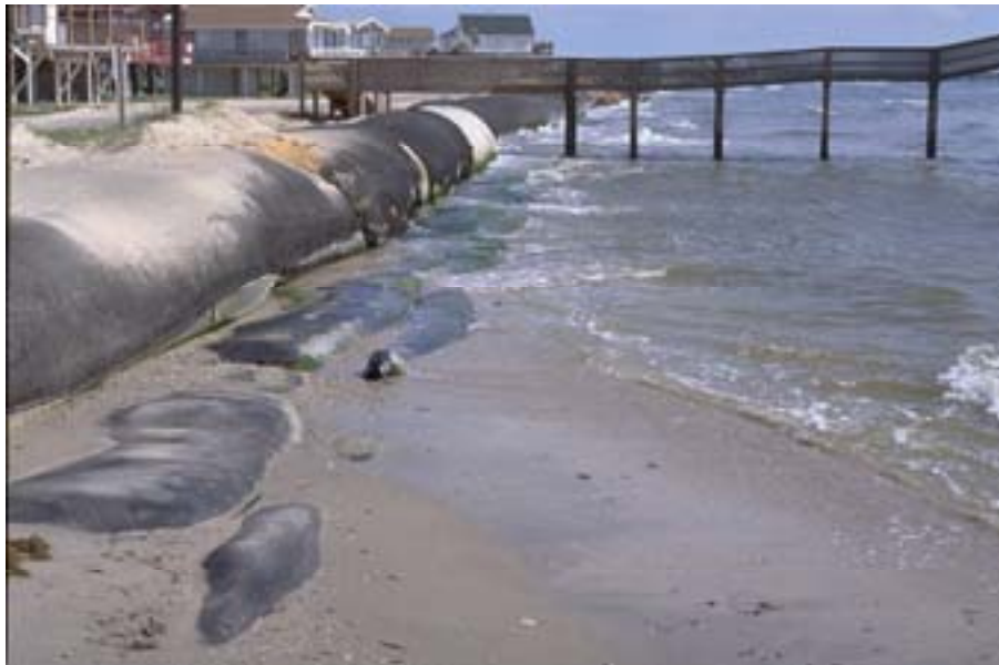
Figure 25. Treasure Island middle geotextile tube on July 19, 2001. Except for a short piece in the foreground this section was completely destroyed in November 2001. Note exposed scour apron and damaged UV shroud. Tube has begun to lose its shape and slump seaward in places.
