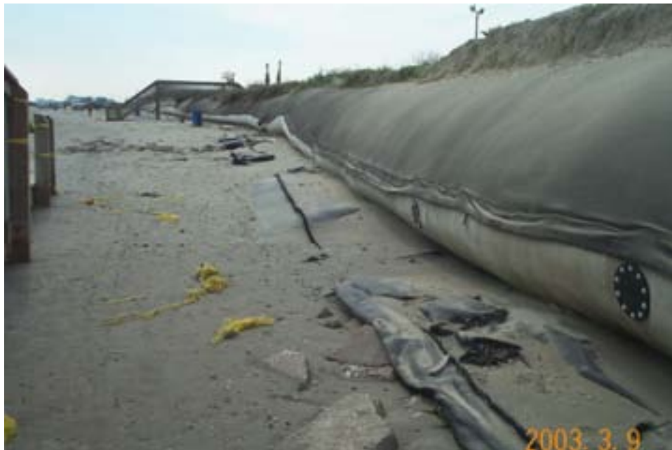
Figure 21. Seaward scour apron exposed and damaged and patched holes in Dellanera geotextile tube on March 9, 2003.
