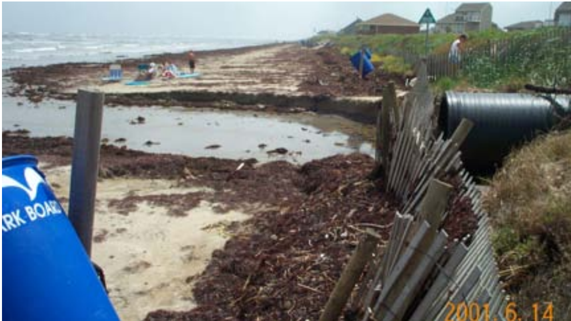
Figure 30. Pirates Beach geotextile tube project on June 14, 2001 after Tropical Storm Allison. Rainfall runoff from Allison flowed through the black street drainage pipe beneath the tube on the right and eroded this channel in the beach.
