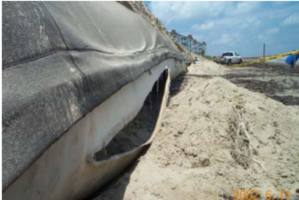
Figure 22. Tear in Dellanera geotextile tube on June 11, 2002. Some have speculated that this hole was the result of vandalism. It has since been patched
