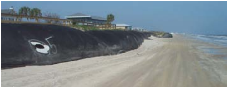
Figure 23. Slumped and collapsed geotextile tube with patched hole near east end of Gilchrist West project (in Caplen) on March 10, 2003. Note completely collapsed section in distance where tube turns seaward.
