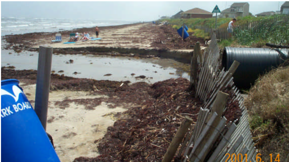
Figure 19. Pirates Beach geotube project on June 14, 2001 after Tropical Storm Allison. Rainfall runoff from Allison flowed through the black street drainage pipe beneath the geotube on the right and eroded this channel in the beach.
