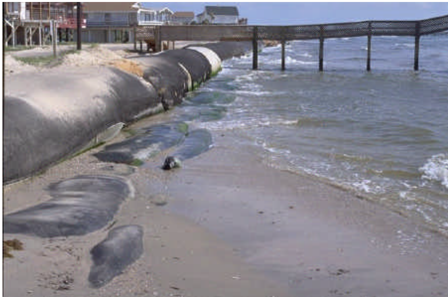
Figure 14. Treasure Island middle geotube on July 19, 2001. Except for a short piece in the foreground this section was completely destroyed in November 2001. Note exposed scour apron and damaged UV shroud.
