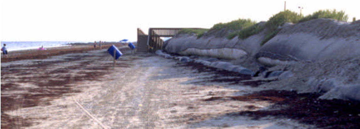
Figure 7. Example of fully exposed geotube front and scour apron at the Dellanera project on Galveston Island, July 18, 2001.
