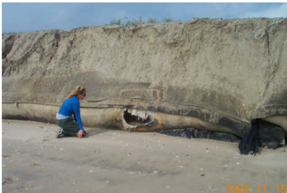
Figure 15. Puncture in Gilchrist West geotube on November 15, 2001.
