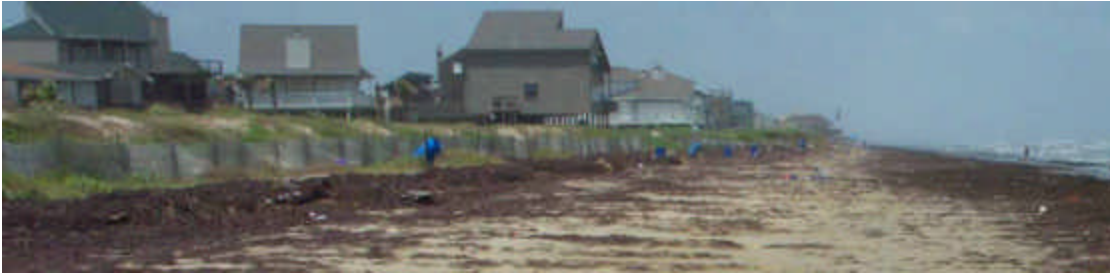
Figure 16. Pirates Beach geotube at GAL01 profile location (see figure 6 for location). This geotube remained covered and vegetated following Tropical Storm Allison. Note sand fence and lack of coppice mound subenvironment.
